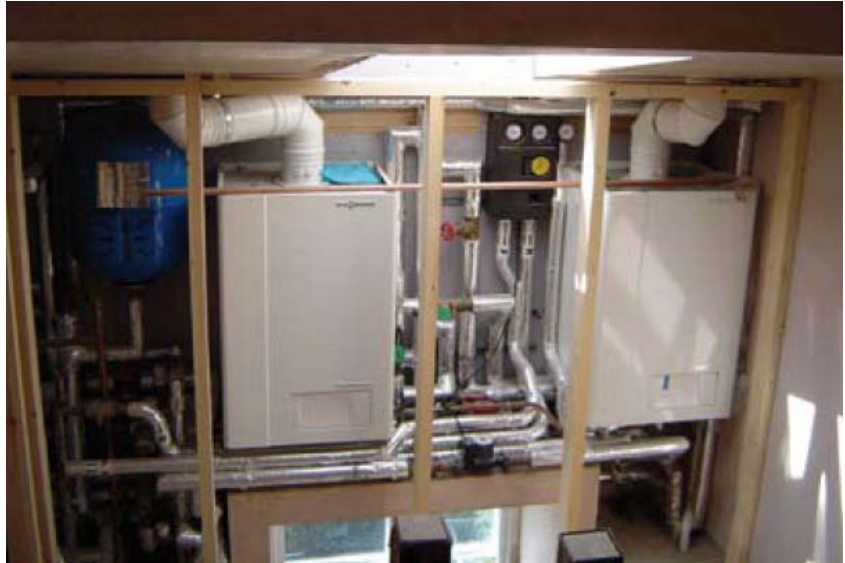
Two communal 26kW condensing boilers provide heating to the whole building
